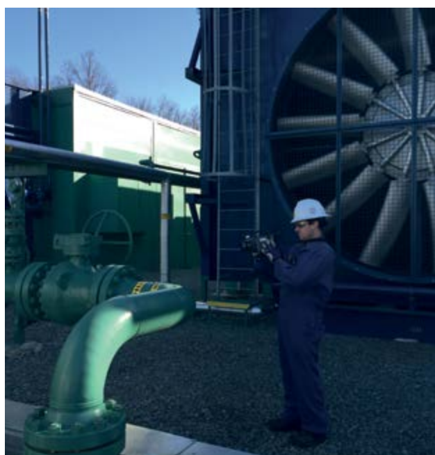
Operator conducting leak detection and repair survey with an optical gas imaging (OGI) camera on one of our Appalachia sites in the USA.
